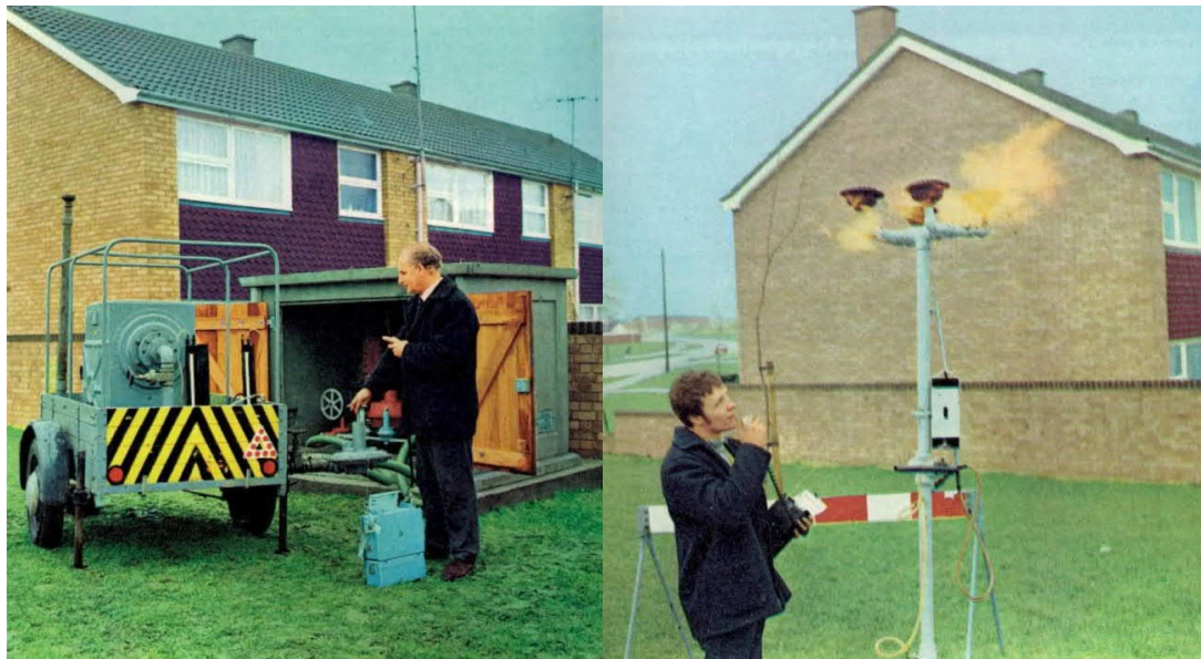
Figure 6.5. Metering in gas (left) and flaring of gas during ‘Turn out’ in the SoGB Region. Source - National Gas Archive.
