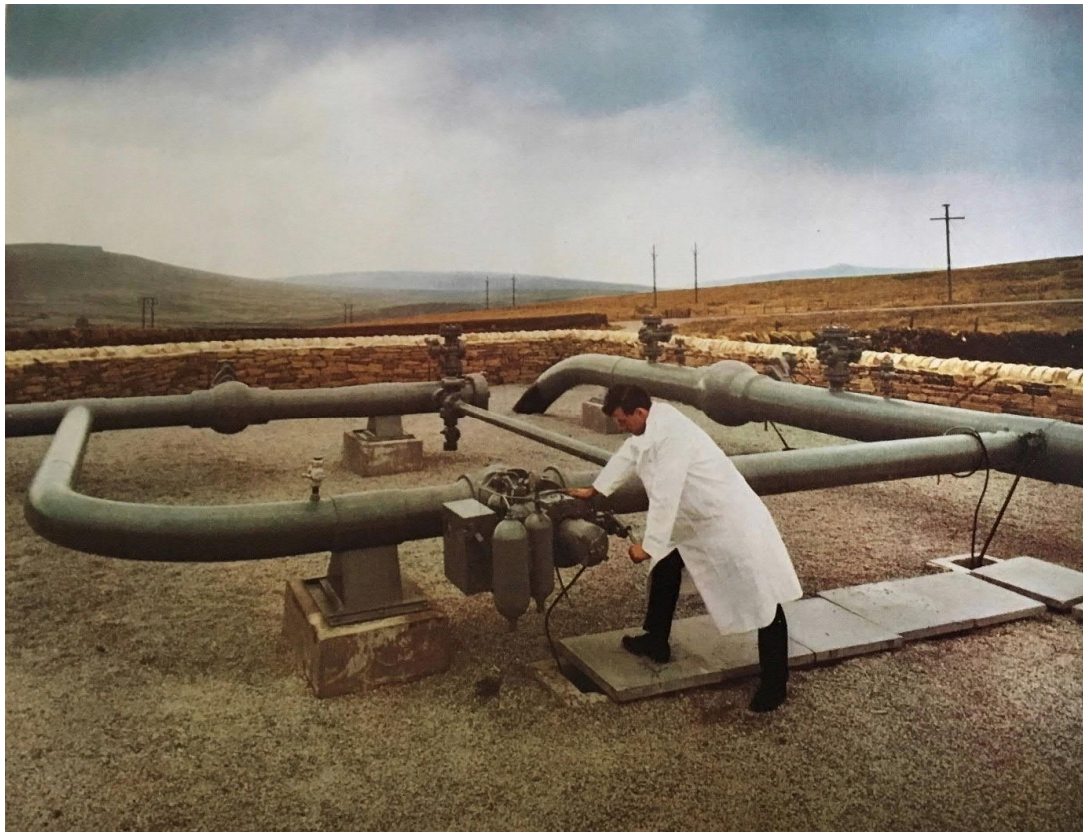
Figure 5.16. The Moscar site in the Pennines where a branch line fed Sheffield from the National Methane Pipeline. Source – Author.
