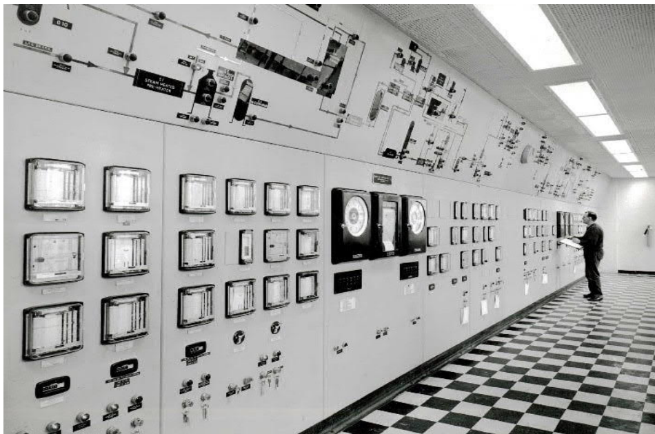
Figure 5.15. Canvey Island Terminal with Methane Princess docked (top) and inside the Control Room (bottom). Source - National Gas Archive.
