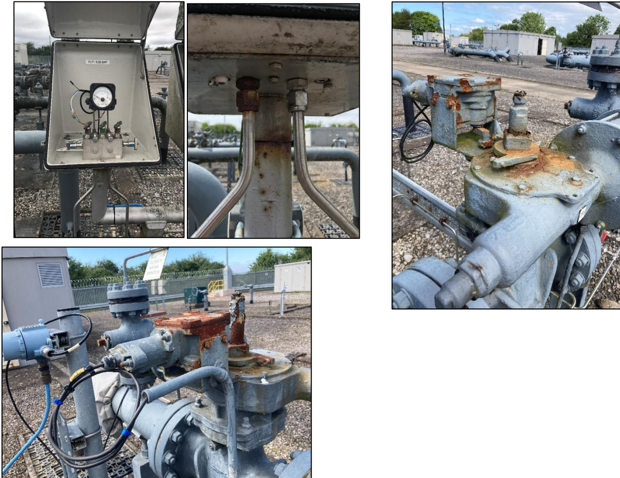
Figure 1 - Yeovil PRS Slam shut Switches & Instrumentation
