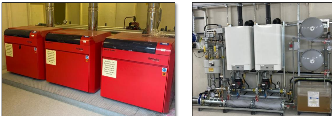
Figure 14 - old, non-condensing boilers, right: new, 2x 90kW condensing boilers
