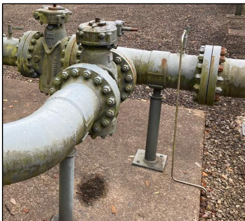
Figure 7 - Original pipe support, unable to inspect between pipe and support
