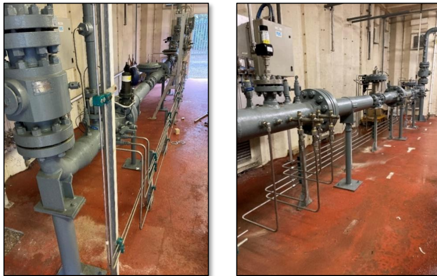
Figure 15 - Left: original, venting flow controller. Right: new, non-venting flow controller
