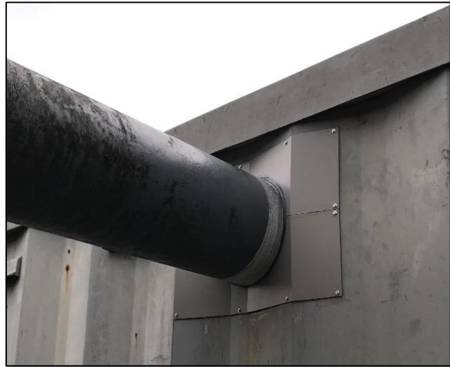
Figure 12 - Assessment carried out, new coating applied to pipework and removable weather guard installed
