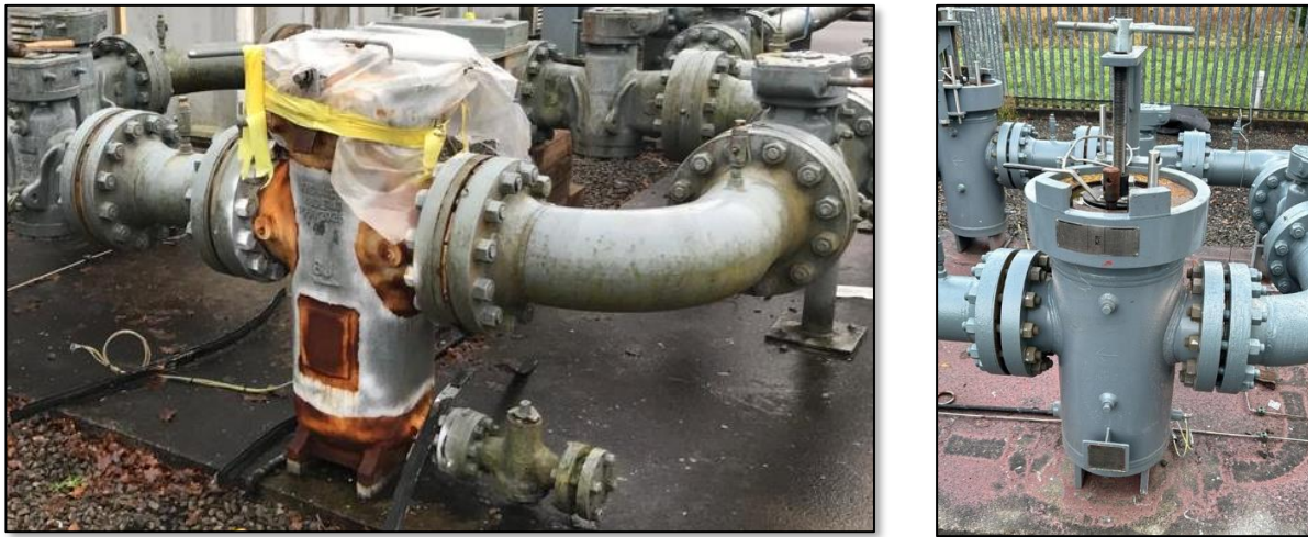
Figure 13 - Old defective filter following inspection (left) and new filter (right)
