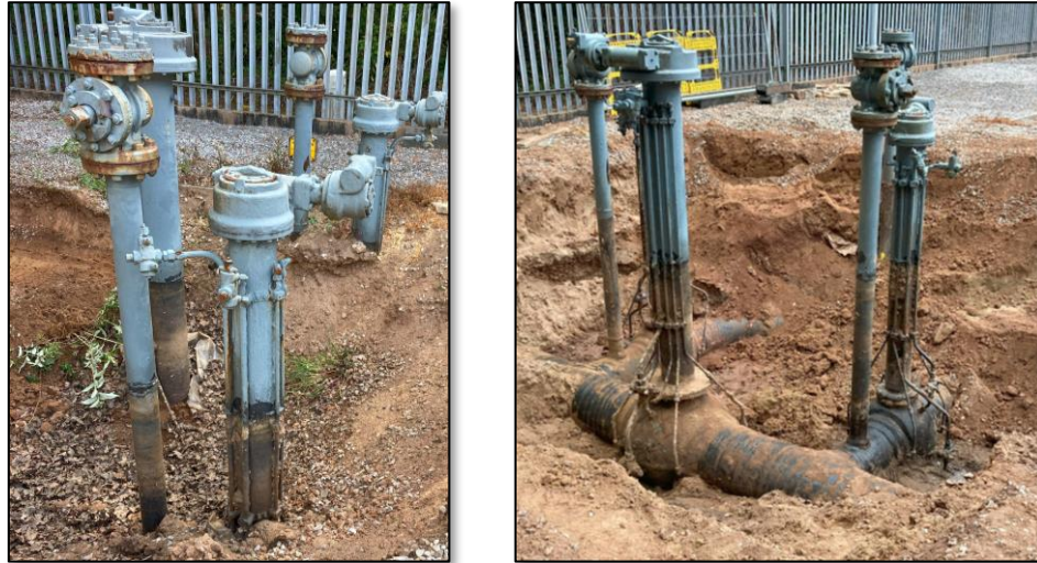
Figure 9 - Removal of a section of compound ground and condition assessment of pipework performed
