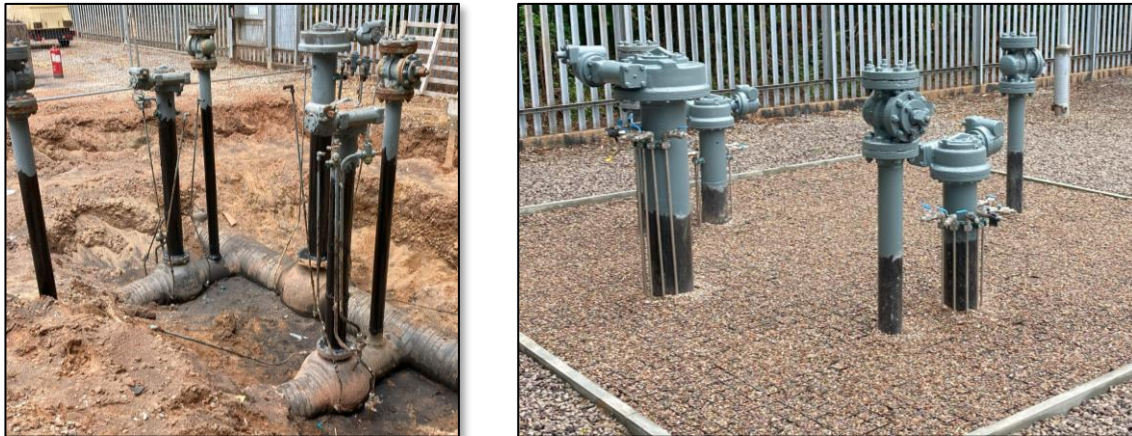
Figure 10 – New multi-component coating system applied to pipework to 500mm above ground level (left) and reinstated with sand and rodent-guard mesh panels to facilitate future inspection (right)
