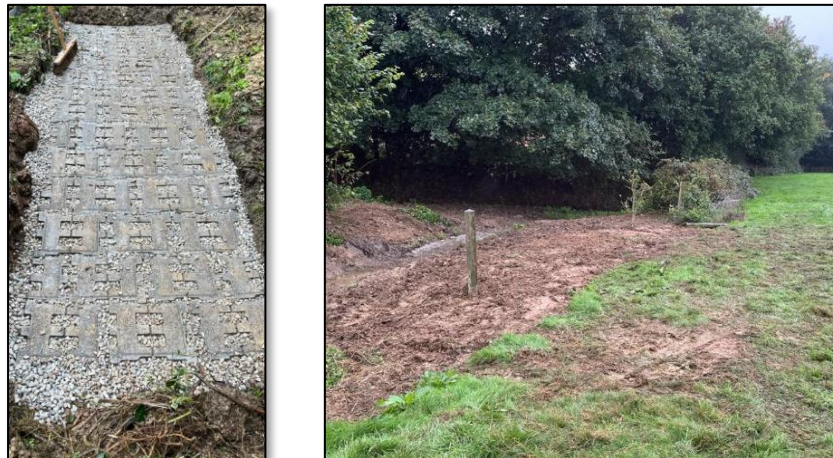
Figure 12 - Picture showing completed project, with cleared vegetation and installed concrete padding over the pipeline
