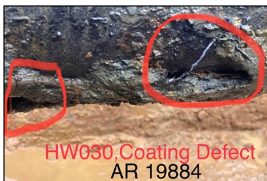
Figure 13 - Coating defect after excavation of the pipe section
