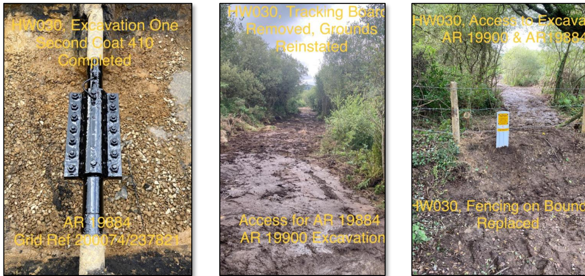
Figure 15 - Completed shell with coating (left), reinstated track (middle) and newly installed fence / marker post (right)
