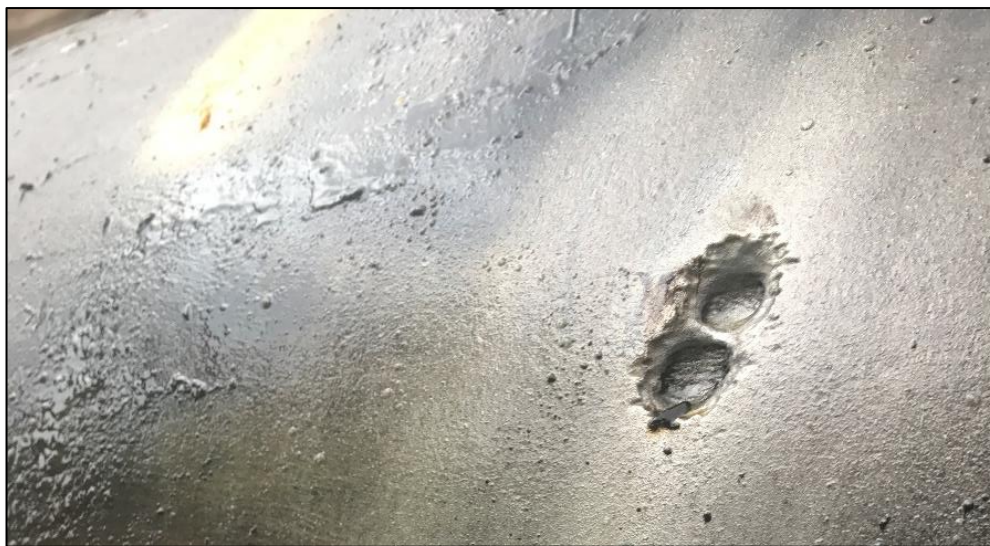
Figure 5 - AC induced metal loss defect (~50% pipeline wall loss), subsequently shelled
